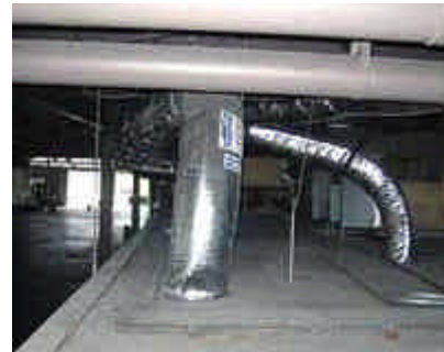
When Payless Insulation moved into its new 46,000-square-foot building earlier this year, the owner couldn’t wait to rip out the existing fiberglass ductwork and install Superior Air Ducts (above and below).
