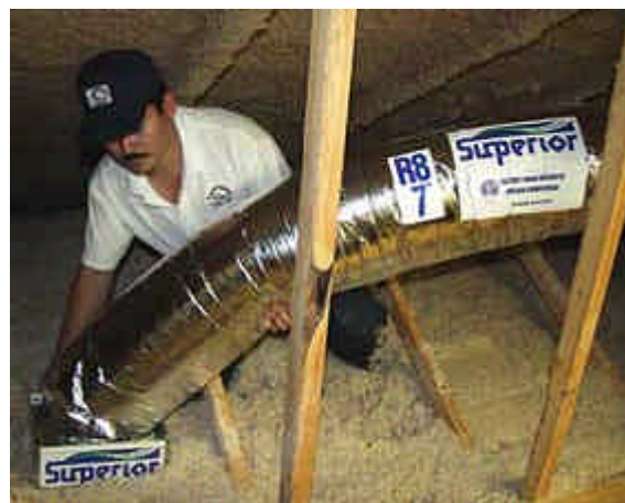
The building's existing metal ducts were cleaned, taped, and sealed, then Superior Air Ducts were installed.
