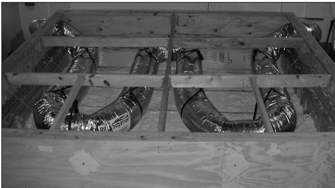
Figure 2. ORNL’s testing lab includes a “simulated attic” installed in a large-scale climate simulator (see the “News Briefs” section of EDU , July 2004). The apparatus was recently used to test the performance of three types of flex duct.
